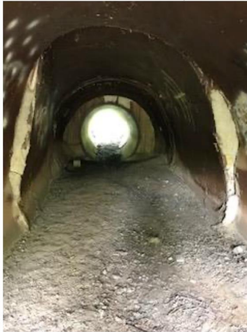
Three Piece Structure: Tank-Tank-Pipe
